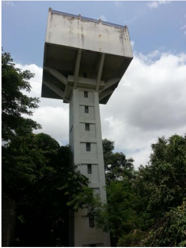
TPH (near Mechanical)
